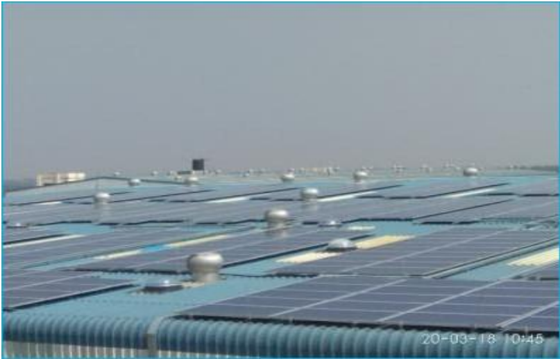
Rooftop Solar at Hosur Plant
