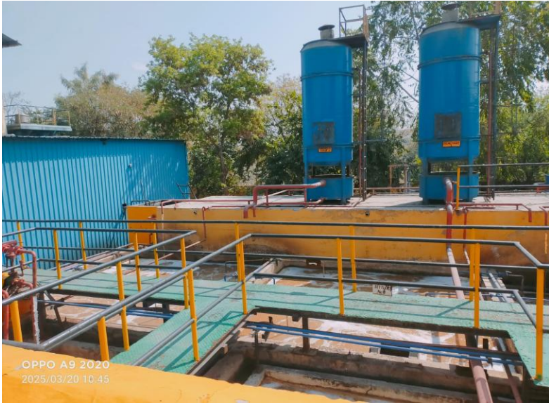
Rainwater Collection inside Bawal Plant Premises
