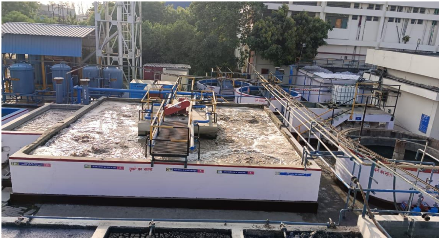
ETP at Jainpur Plant
