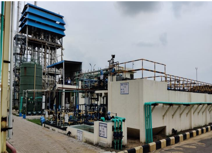
ETP at Sayakha Plant
