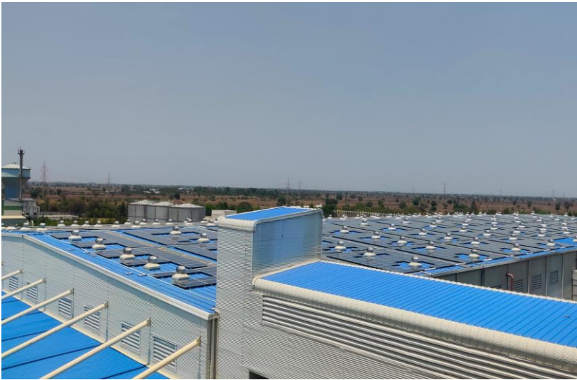
Rooftop Solar at Sayakha Plant
