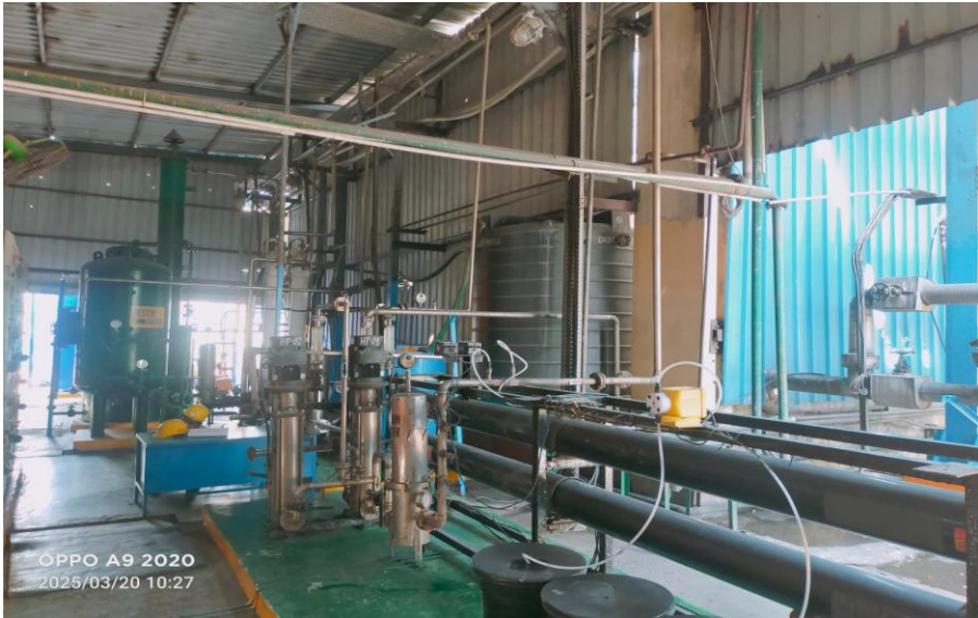
Effluent Treatment at Bawal Plant
