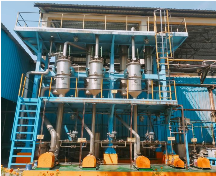
ZLD at Bawal Plant
