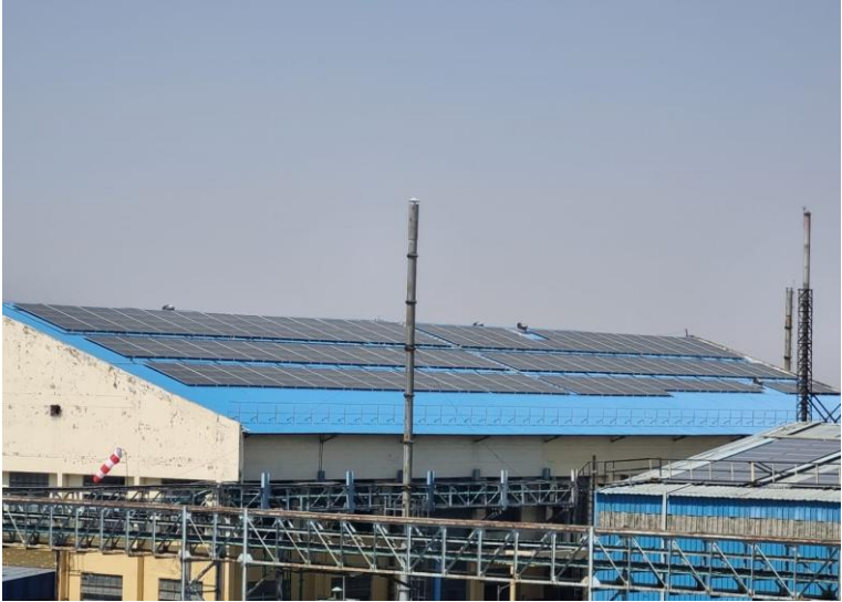
Rooftop Solar at Jainpur Plant
