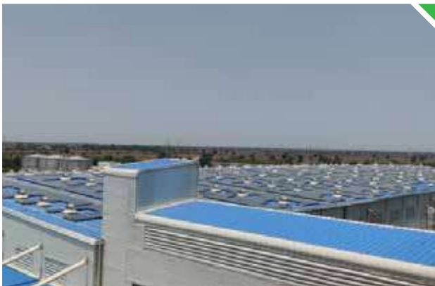
Solar Energy - Sayakha Plant
